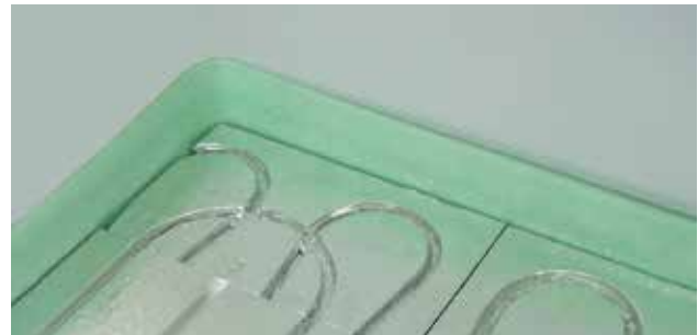
Start of laying PRINETO U-turn elements in a corner of the room.
